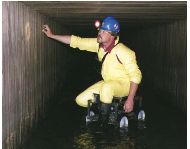
HK Sr. Service Technician, Kim Krebs, creeps along a specially made cart, while inspecting the wooden structure of an old storm sewer beneath the streets on the east side of Des Moines.
